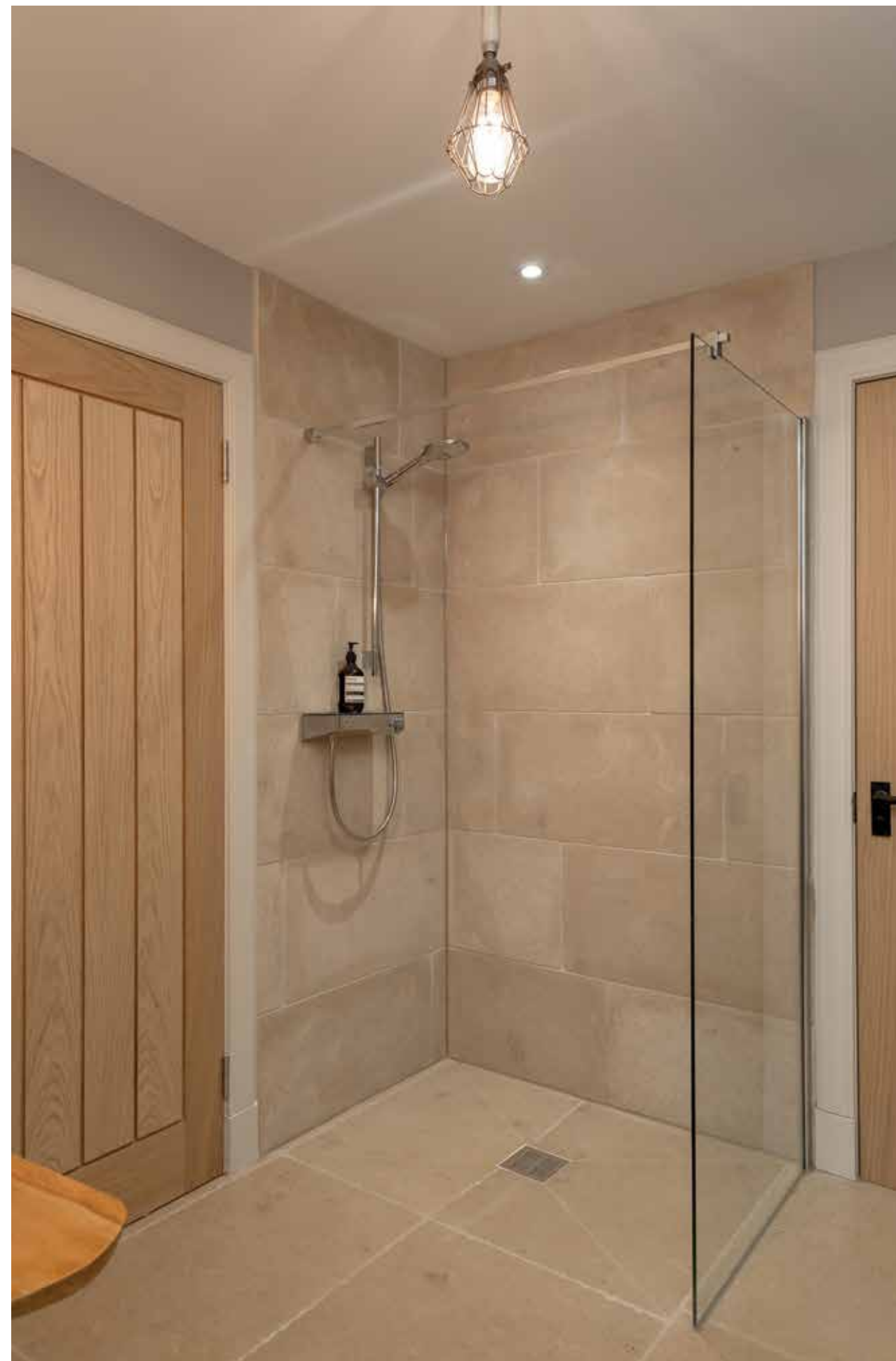
Left: A wetroom panel was installed to protect the rest of the bathroom from splashes and allows full access from the front of the shower.
